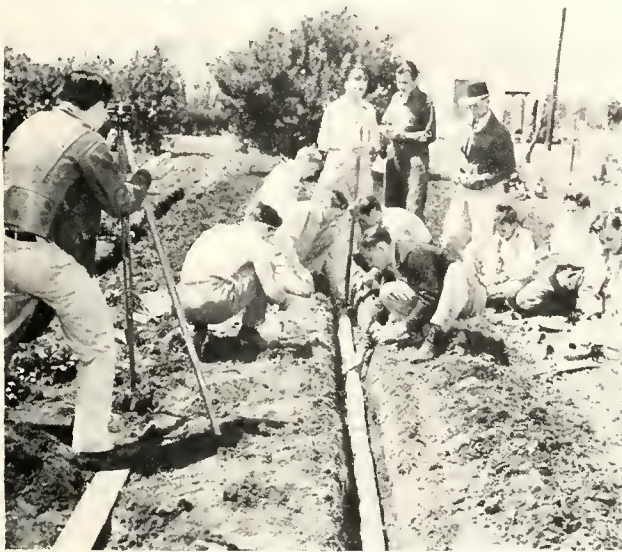
A group of F.F.A. members learn to lay tile for drainage. Under the direction of the teacher of vocational agriculture they receive instruction in farm mechanics.
